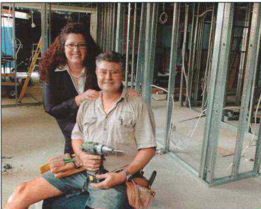
ALMOST THERE: Stephanie Shepherd massages carpenter John Durand, on the job at Sofitel.
